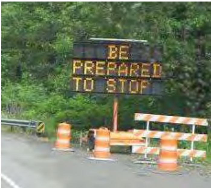
Example of using a message board to educate drivers
