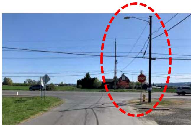
Luminaire oriented towards side street
